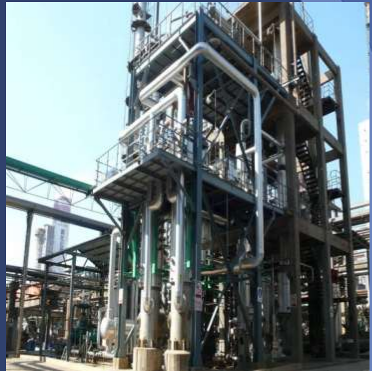
3500 t/a DEMO plant
