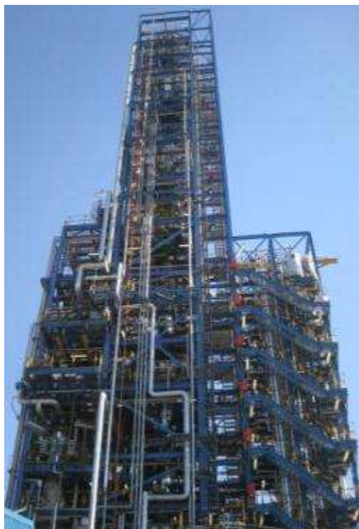
Reactor Demonstration Facilities in South Africa Slurry Phase Design Reactor for Hydrocarbon Synthesis (400bpd) and Catalyst Testing Reactor (5bpd))
