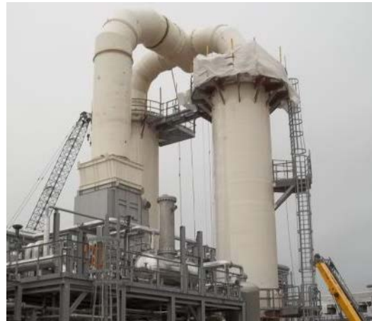
Steam methane reformer
