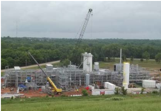
View of GTL plant from landfill site
