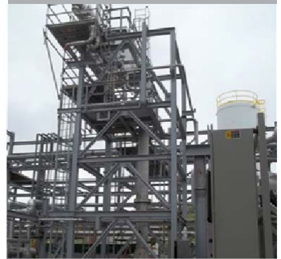
CO 2 wash column
